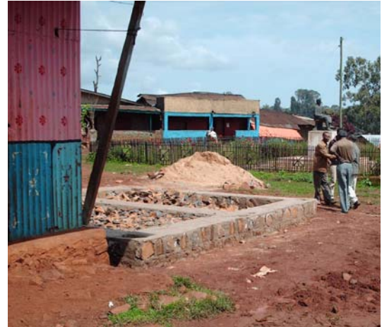
This is the site for an iron store for income generation similar to those in Mettu.
