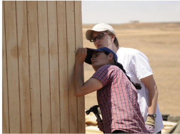
Lorentino's neighbor Elena helps Bekah nail the walls together at the corner.
